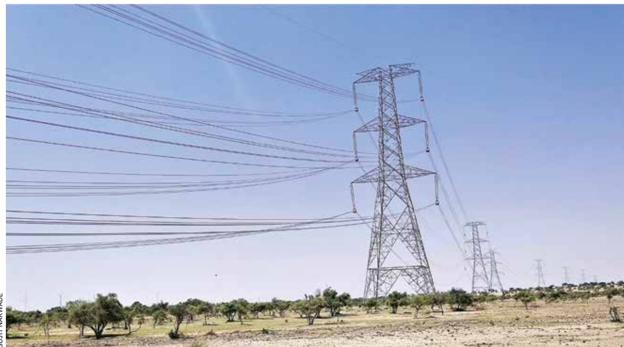
New high voltage power lines are coming up in the Thar area despite a stay order by National Green Tribunal
